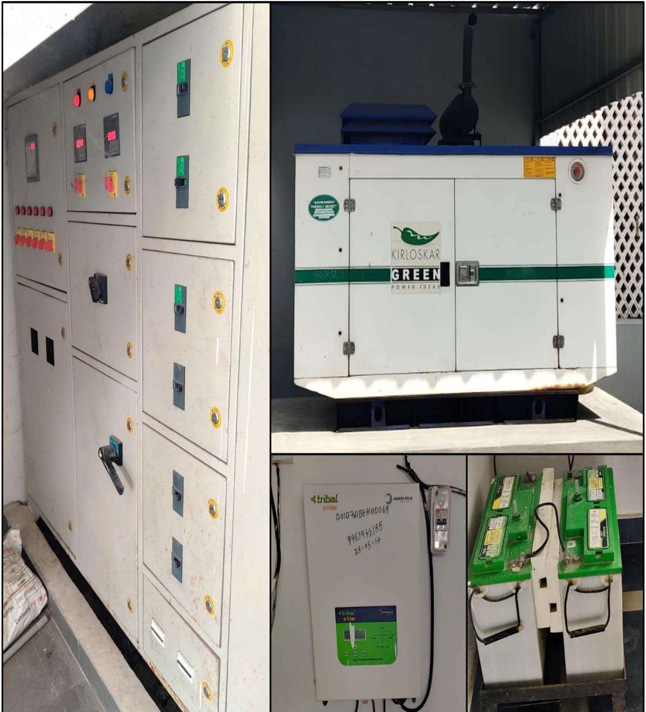
Power Room, Generators and UPS Room well maintained in the St. Ann's College for Women, Guntur, Andhra Pradesh
